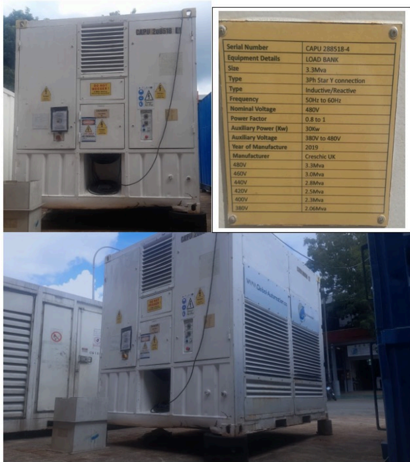
LOAD BANK 3.3 MW
